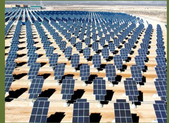
Large photovoltaic farm
